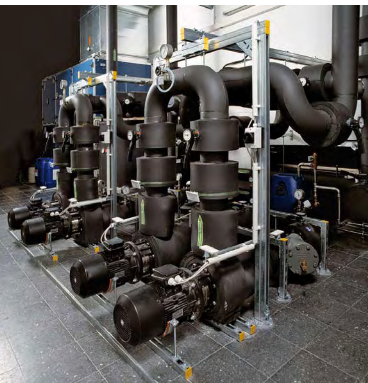
The central transmitter cooling system in Munich's Olympic tower.
